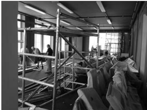
Work in progress on the transformation of the former Clapham Library into Omnibus, Clapham's first arts centre.
